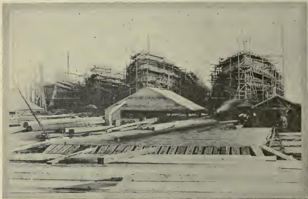
FOUR WOODEN SHIPS IN COURSE OF CONSTRUCTION AT THE YARD OF THE GRAY'S MOTOR SHIP CORPORATION, ABERDEEN, WASHINGTON.
